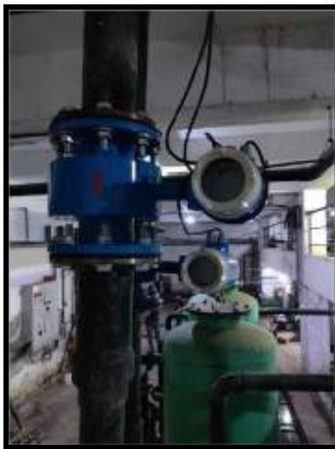
Photograph of Electromagnetic flow meter provided at Flushing plumbing line and treated water supply line to green area
